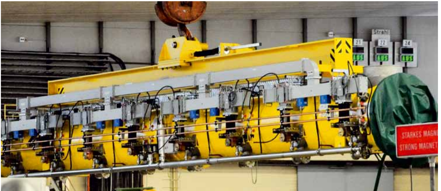
Figure 2 RF waveguide distribution and accelerator module during transport
