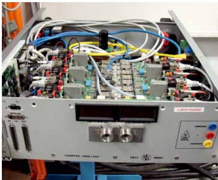
Figure 3 200 A choppers. There are four 50 A power modules plus two identical ones for redundancy.
