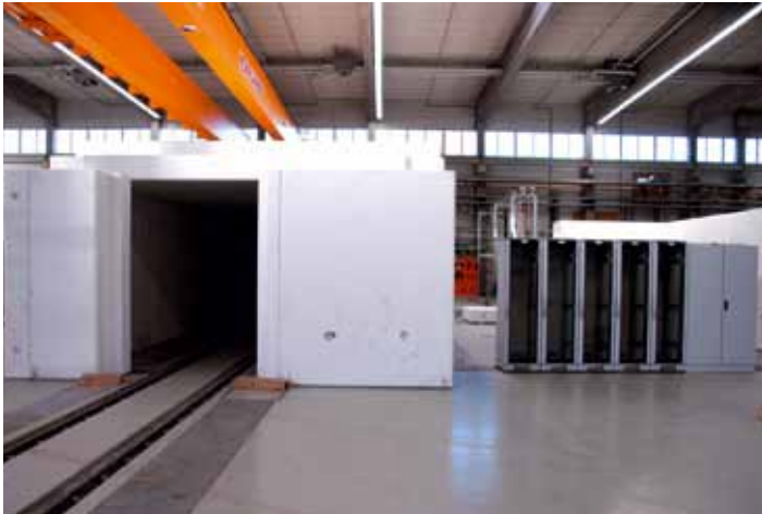
Figure 2 Radiation protection elements of one of the cryomodule test stands inside the AMTF
