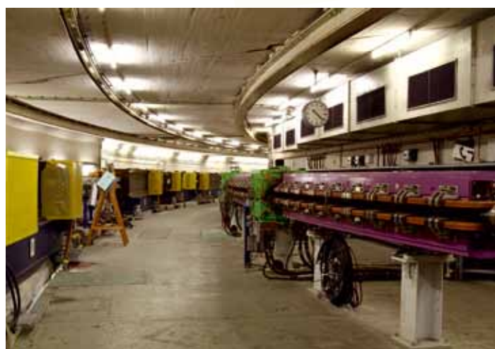
Figure 2 View of the DESY tunnel, DESY II is on the right.
