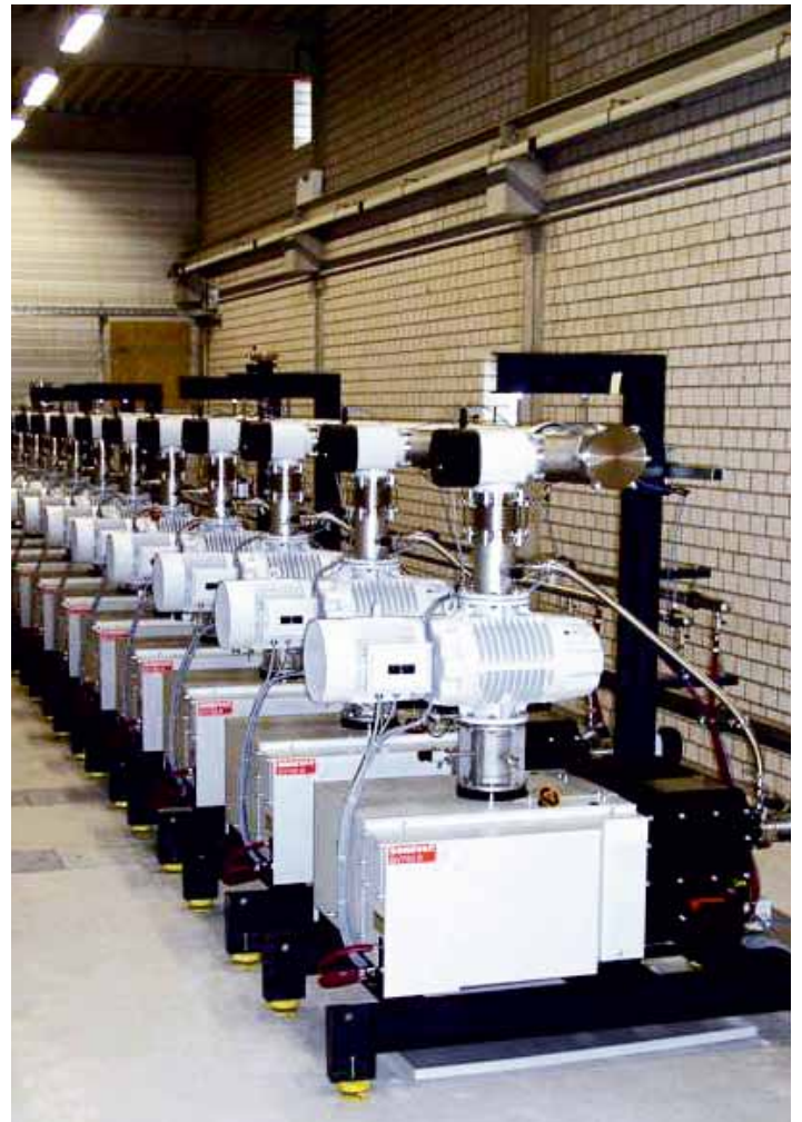
Figure 3 One of the two AMTF helium pump sets
