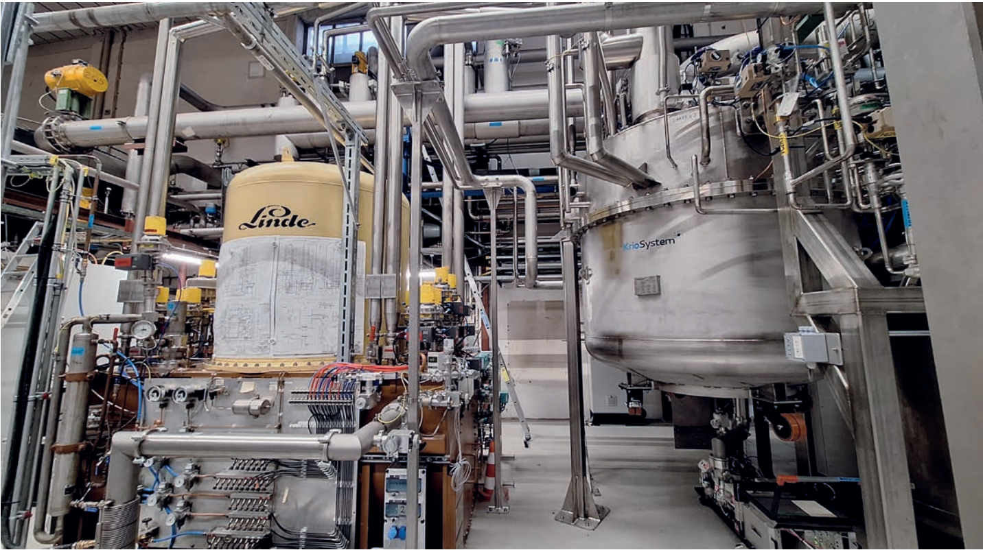
Figure 2 The cryogenic plant and distribution box for the SUNDAE1 test stand
