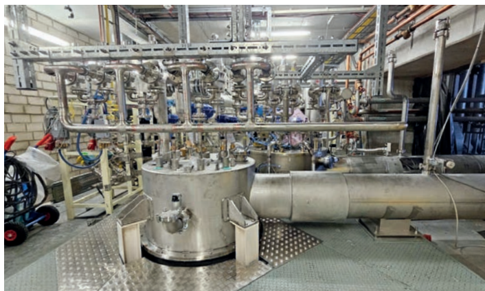
Figure 1 Top: Two-valve configuration in the main accelerator tunnel (lower left corner) with complex vessel piping. Bottom: Cryogenic feedbox in the injector building.
