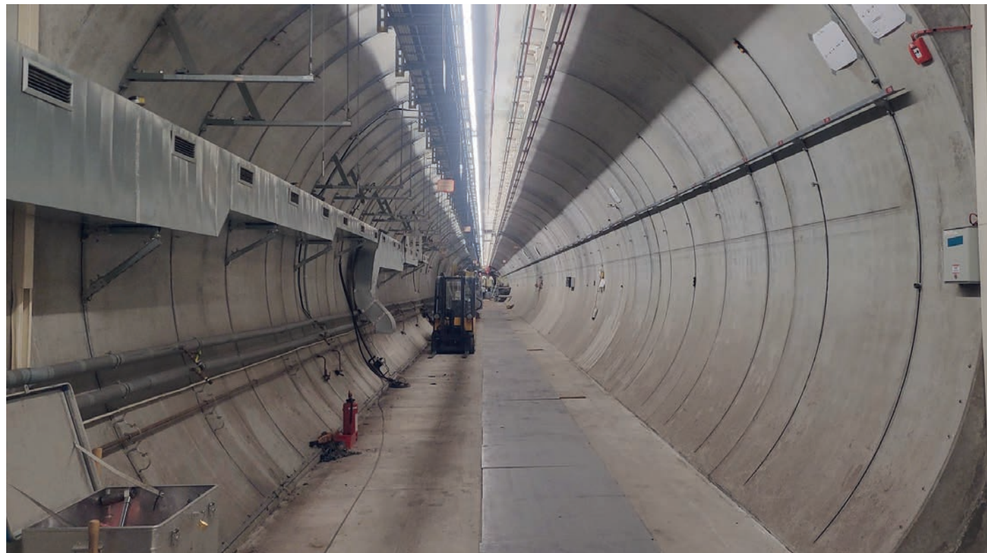
Figure 4 View into the emptied FLASH1 tunnel in autumn 2024, providing about 120 m of space for a new electron beamline, undulators, laser and photon beamlines and all the related infrastructure around.
