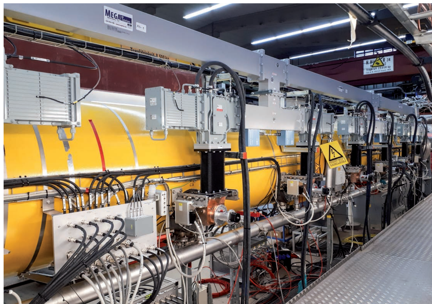
Figure 1 One of the two new superconducting accelerator modules (in yellow) installed in the FLASH tunnel replacing two old ones.
