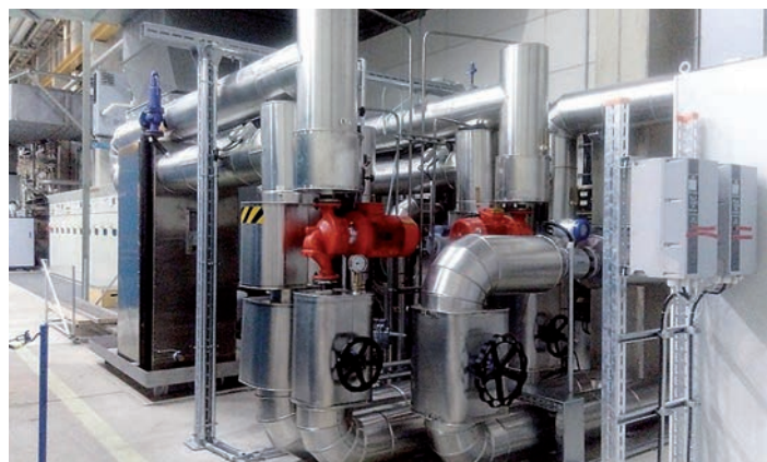
These heat exchangers in the DESY cryo plant feed heat into the DESY heating network.
