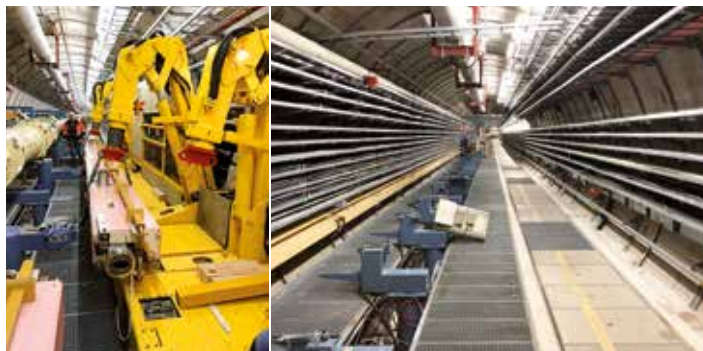
Figure 1 Left: Dismantling of the HERA accelerator in the ALPS II area. Right: The empty tunnel segment in autumn 2018.
