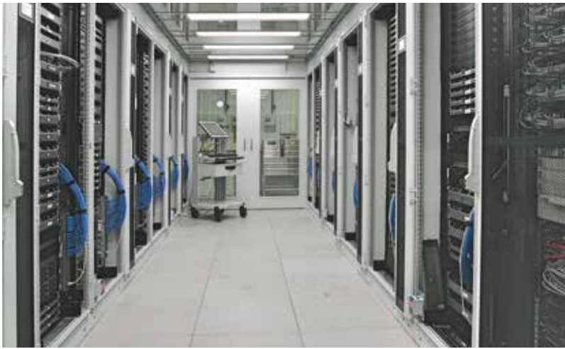
Figure 1 New cold aisle containment inside the RZ1 data centre at DESY in Zeuthen
