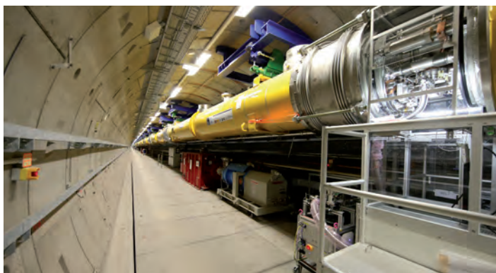
Figure 1 Accelerator modules installed in the linear accelerator section L3. Only some of the 59 modules that were put in place by the end of 2015 are visible. The continuous string of modules at the end of 2015 exceeded 400 m.
