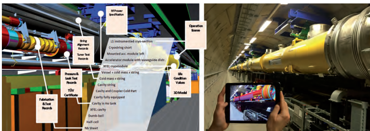
Figure 1 Digital and physical accelerator facility together with examples of the content of the configuration database
