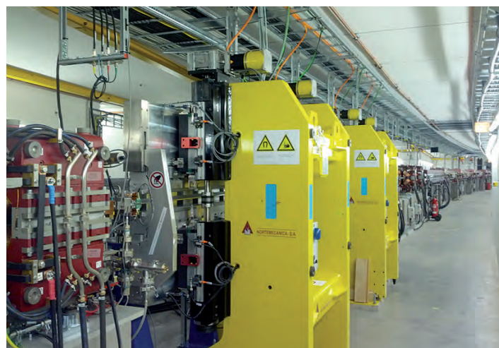
Figure 1 View into the accelerator tunnel in the extension section North (PXN) after installation of the two new undulators PU64 and PU65
