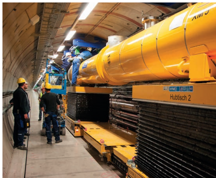
Installation of one of the first accelerator modules in the tunnel of the European XFEL by workers of the DESY-led Accelerator Consortium.
