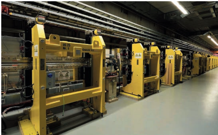
The 30 m long undulator in the FLASH2 FEL line, consisting of 12 segments, which produces the FEL radiation.
