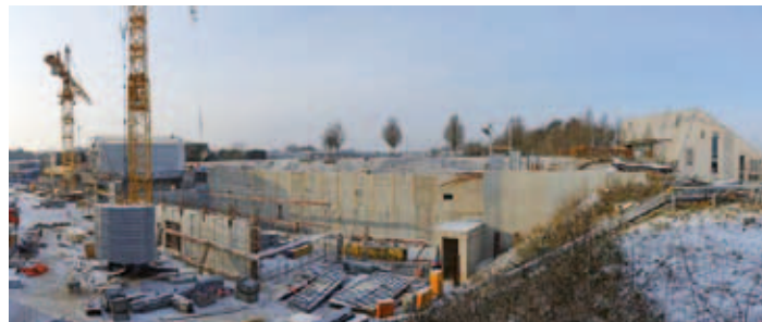
Figure 4 Construction work along the FLASH tunnel for the new FLASH2 undulator beamline
