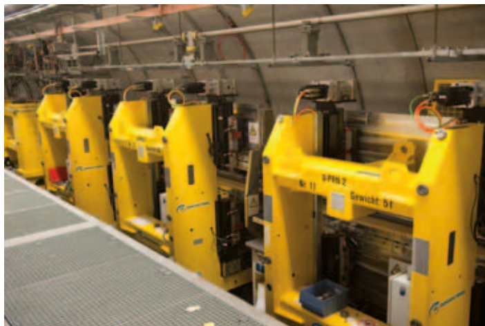
The sFLASH undulators in the FLASH accelerator tunnel
