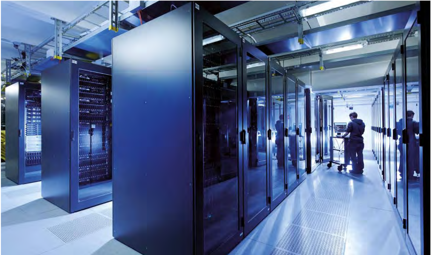
Computer farm for the National Analysis Facility (NAF) and the Tier-2 facility
